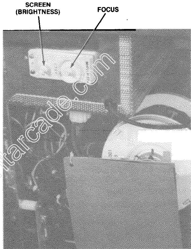
Figure 2 Adjustable Controls on High-Voltage "Cage"
